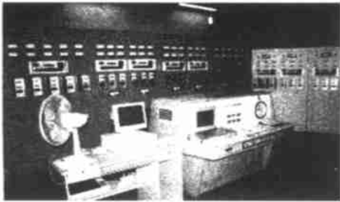
(b) The control equipment
